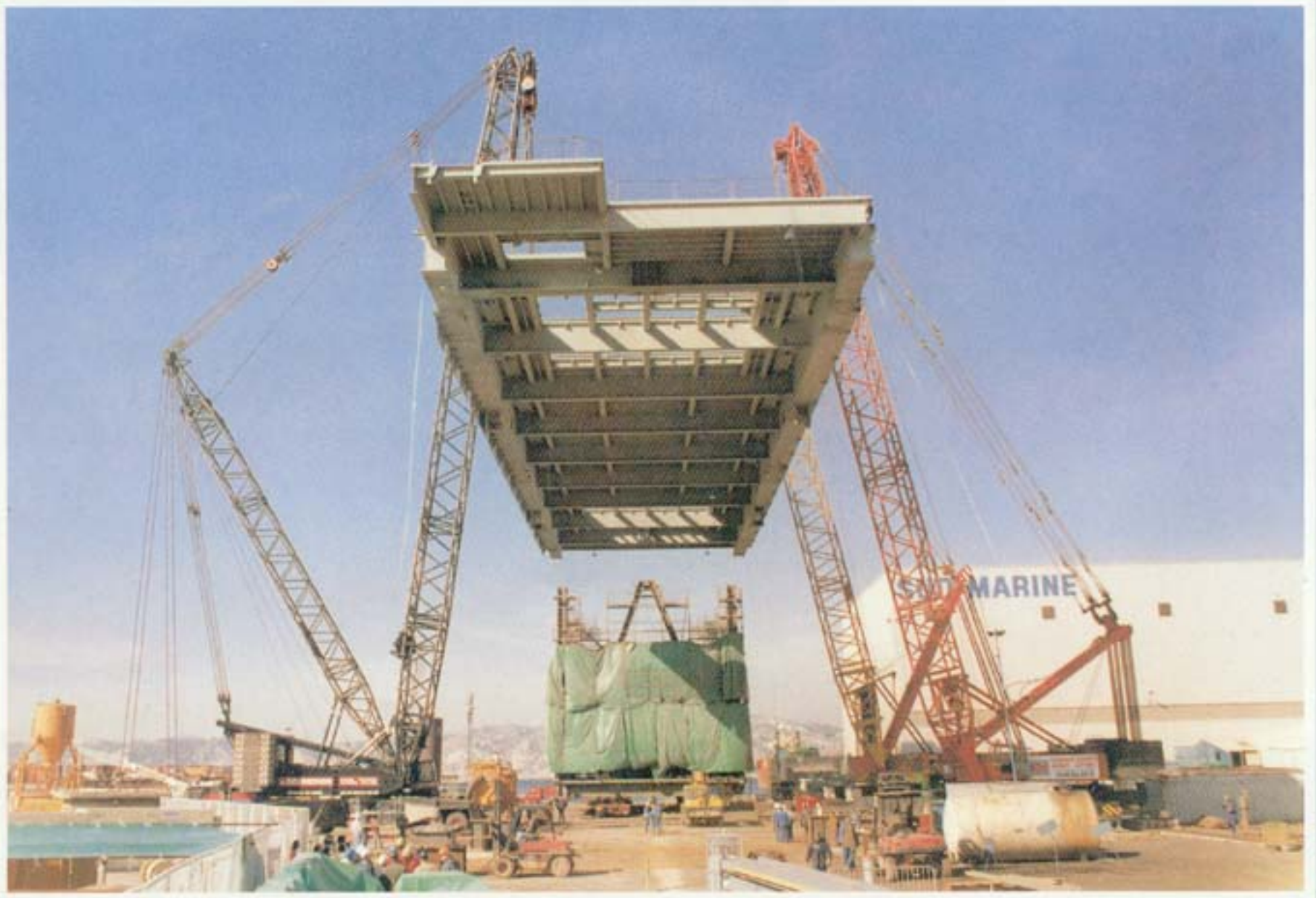
By order of Sud-Marine - France we have done the load-off of several modules with weights of 700 tons with destination Statoil Norway.
